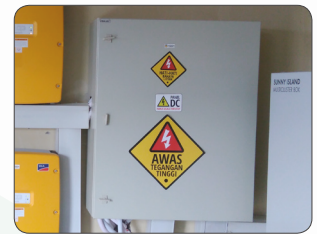
Panel Distribusi DC
